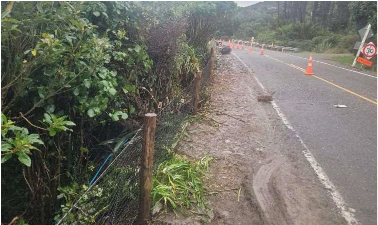
New section of penguin protection fence at Limestone Creek being installed by Westreef
