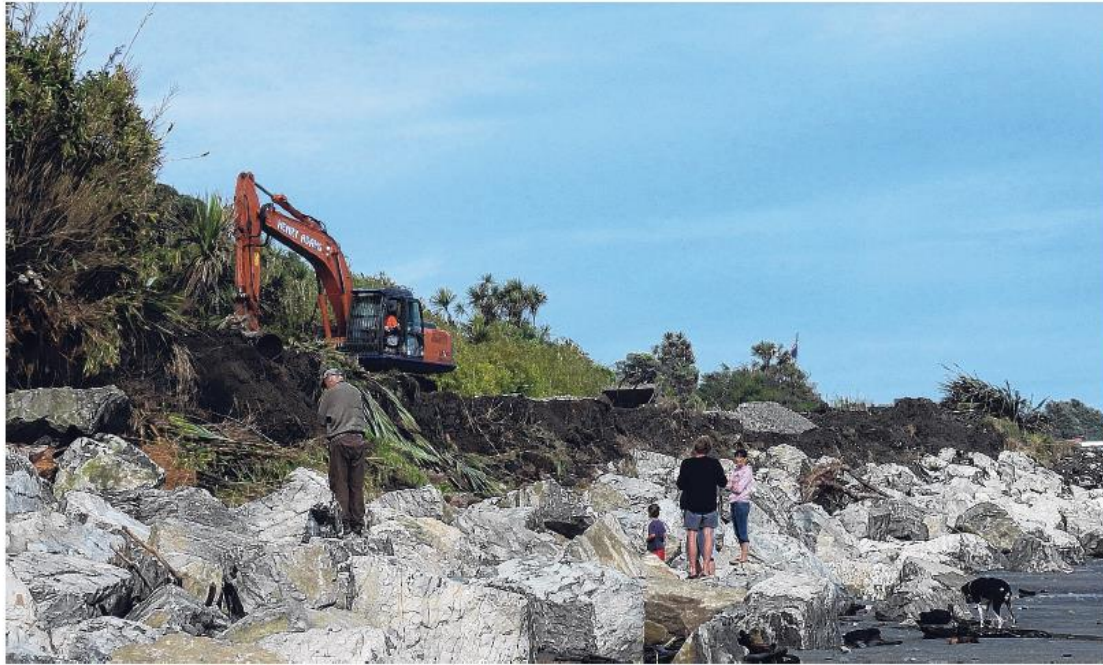
Locals watch on as a digger works to clear vegetation and form an access road from behind Revell St properties to allow emergency rock protection works to be carried out. PHOTO: JANNA SHERMAN
